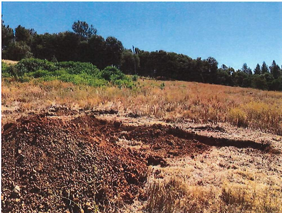
Photo No. 14 View looking southeast at Soil Profile Test Pit TP6. Downslope limit of lush vegetation in Field A is in upper left (photo date 8/6/2020).
