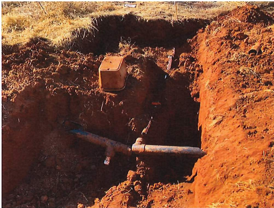
Photo No. 2 Distribution piping exposed in LF1 at the northern margin of Field O. View is looking approximately along contour to the southwest (photo date 8/6/20).
