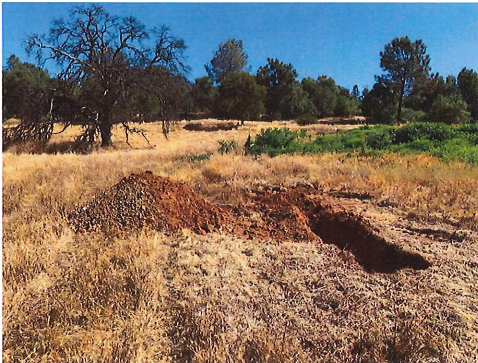
Photo No. 13 View looking northeast at Soil Profile Test Pit TP6. Downslope limit of lush vegetation in Field A is in upper right (photo date 8/6/2020).
