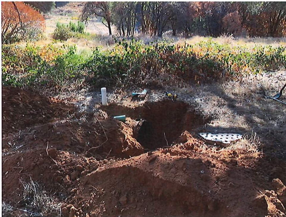
Photo No. 5 View looking east (downslope) at the southwestern portion of Field B and excavation LF2, exposing the end of an infiltrator (photo date 8/7/2020).
