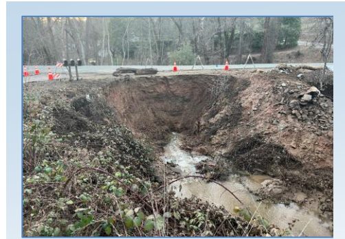
Failed Drainage Culvert on Newtown Road in Placerville.
