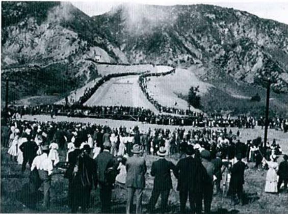
The Los Angeles Aqueduct, carrying water from the Owens Valley, helped the city grow from a population of 214,000 in 1905 to 3.8 million today.
