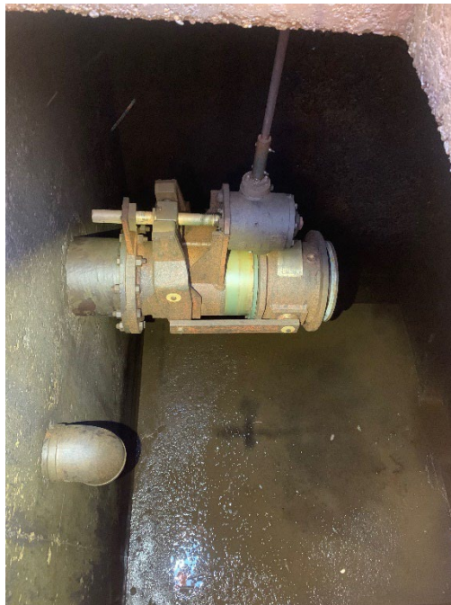
Inspect, Resurface and Lubricate Buckeye Conduit Valve – 8 Labor Hours | Specialty Contractor, Safety Equipment
