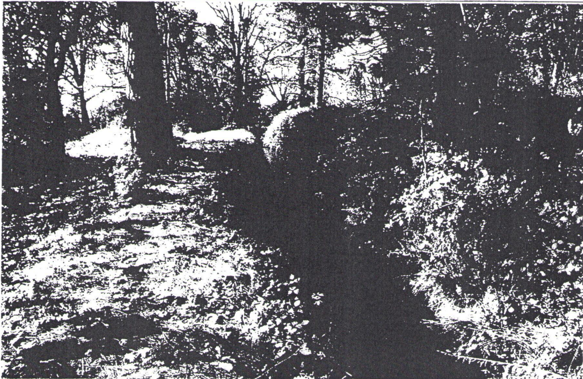
LN 06-11-25: View S70W showing portion of the Georgetown Divide Ditch (gunite-lined) that will be piped as part of the proposed Greenwood Lake WTP project.
