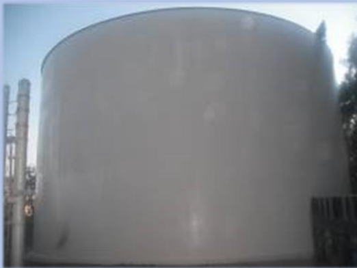
Spanish Dry Diggins Storage Tank
