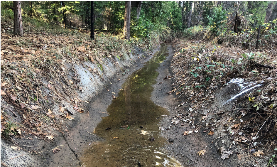
Lined canal section that sustained damage and was repaired during the Treated Water Line and Canal Reliability Project
