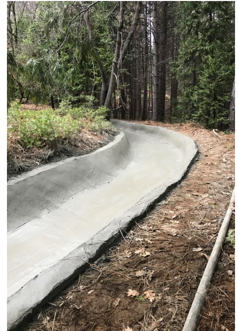
BEN|EN replaced approximately 1,350 linear feet of 4-inch treated water line in Kit Fox Court and Angel Camp Court and improved the main ditch by lining approximately 2,500 linear feet of the ditch with gunite
