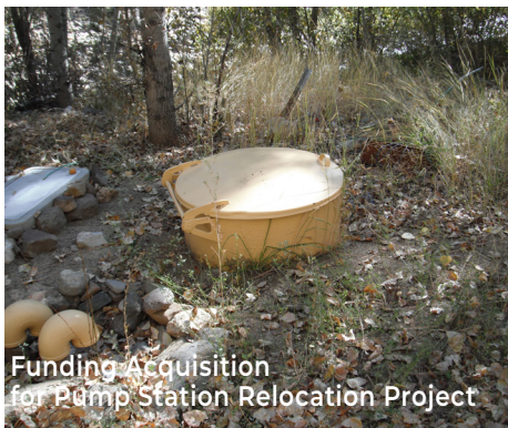
Wastewater Treatment Ponds
