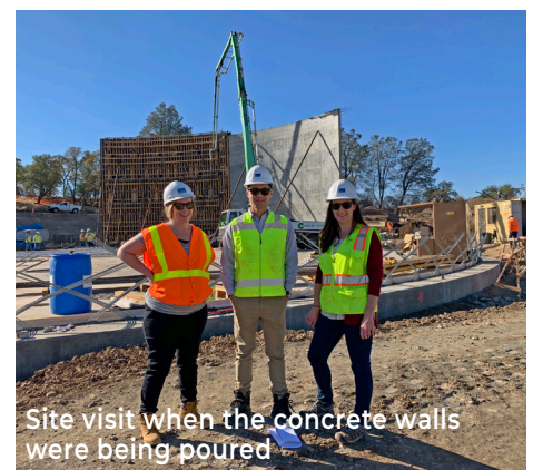
Verdera North Tank #3 and Pump Station
