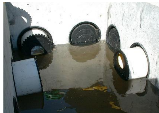
Diverter Caps used to alter flow of effluent.
