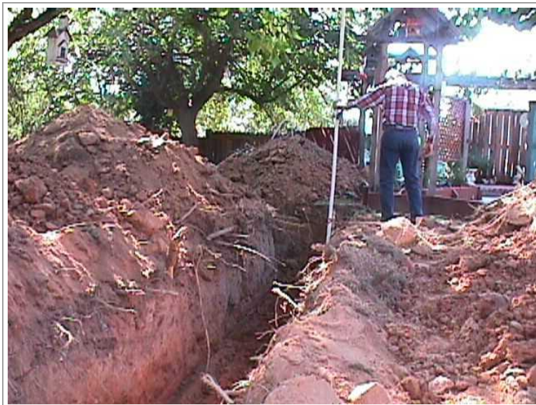
To determine the level of the trench bottom, this contractor is shooting the grade.
