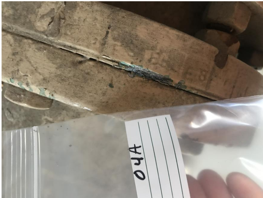
View of asbestos containing gasket.
