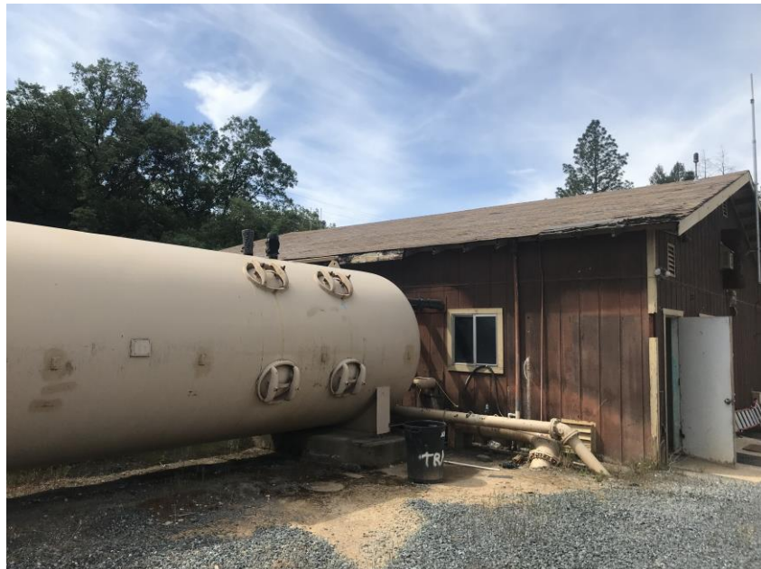
View of one of three filter tanks and Pump house.
