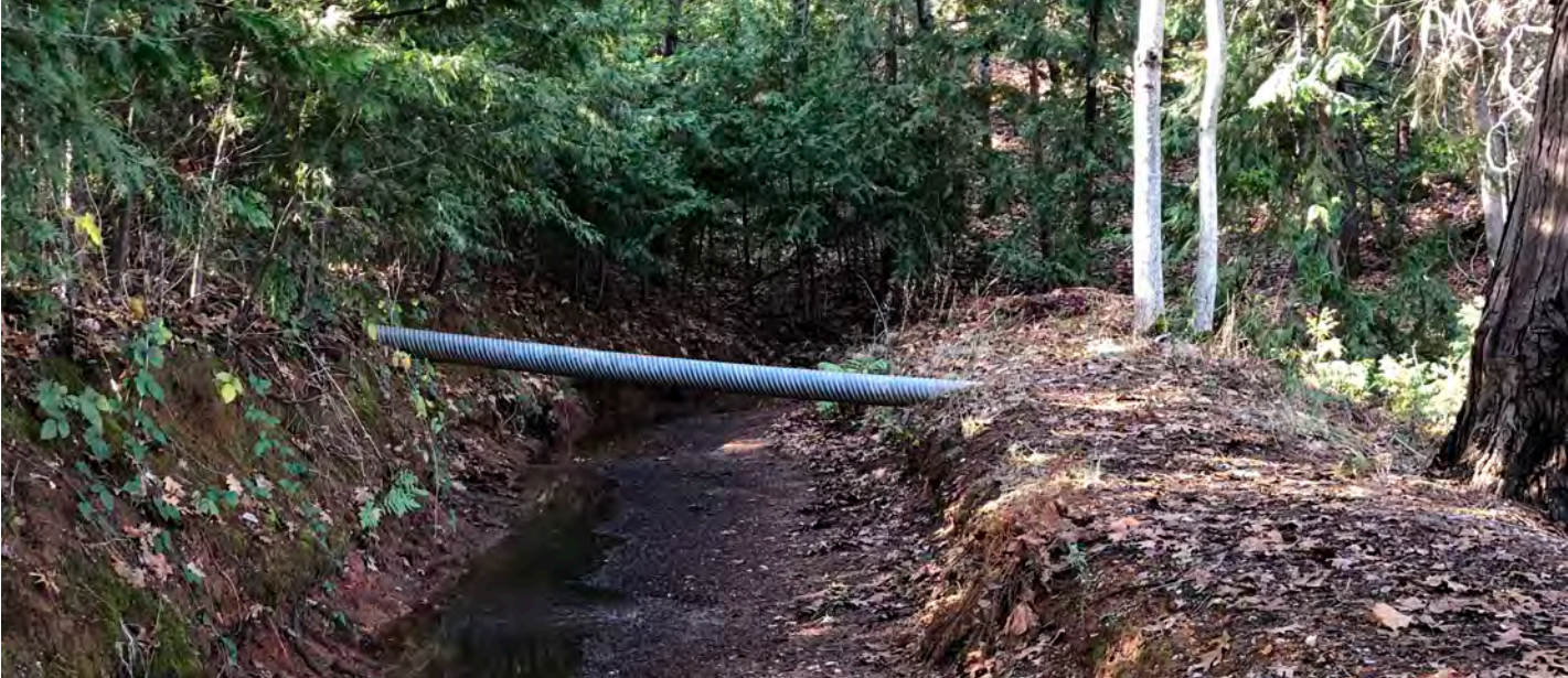
2018 Treated Water Line and Canal Reliability Project – Georgetown Divide Public Utility District
