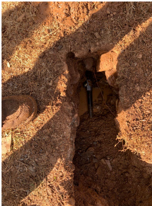
Service Line Repair – 8 Labor Hours | Flat Bed, Vac Trailer, Service Trucks, Hand Tools, Loader
