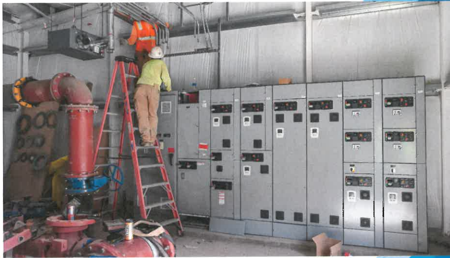
Electrical Control Panel in the Raw Water Pump Station Building
