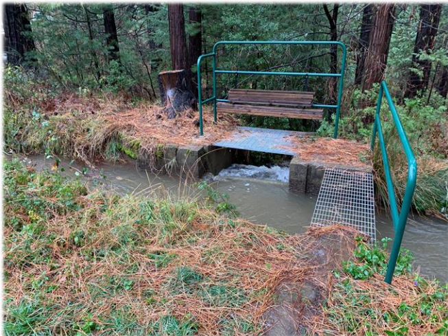
Balderstone Waste Gate
