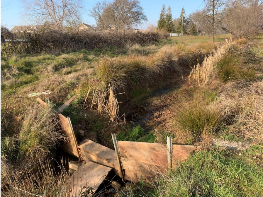
Pilot Hill Ditch Prior to Repair
