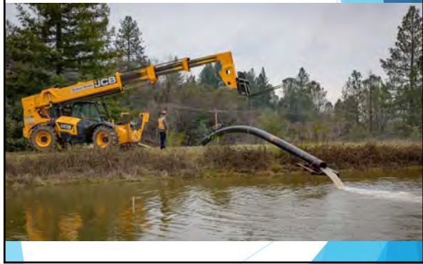
Raw Water Bypass Line
