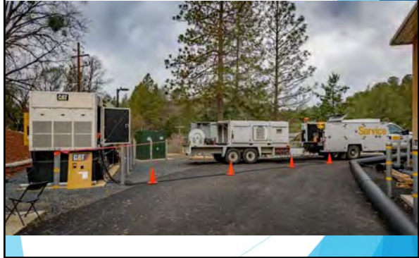
Testing Standby Generator
