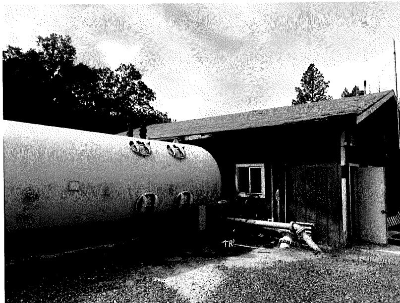
View of one of three filter tanks and Pump house.
