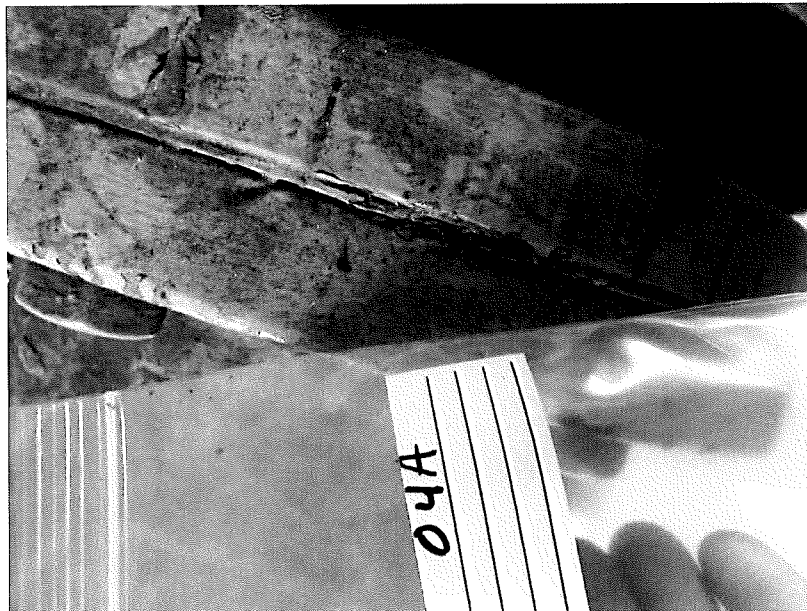
View of asbestos containing gasket.
