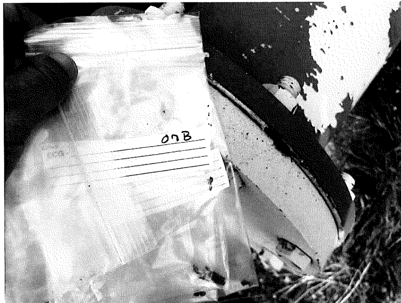
View of asbestos containing gasket.
