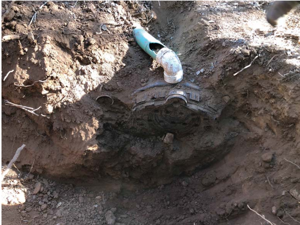
Photo No. 7 Southwest end of Field B, Row 4 infiltrator exposed in excavation LF2. (photo date 8/7/2020).
