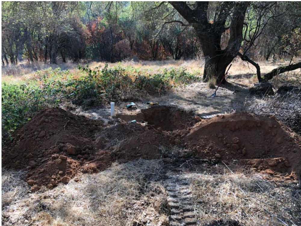
Photo No. 6 View looking southeast at the southwestern end of Field B and excavation LF2 (photo date 8/7/2020).
