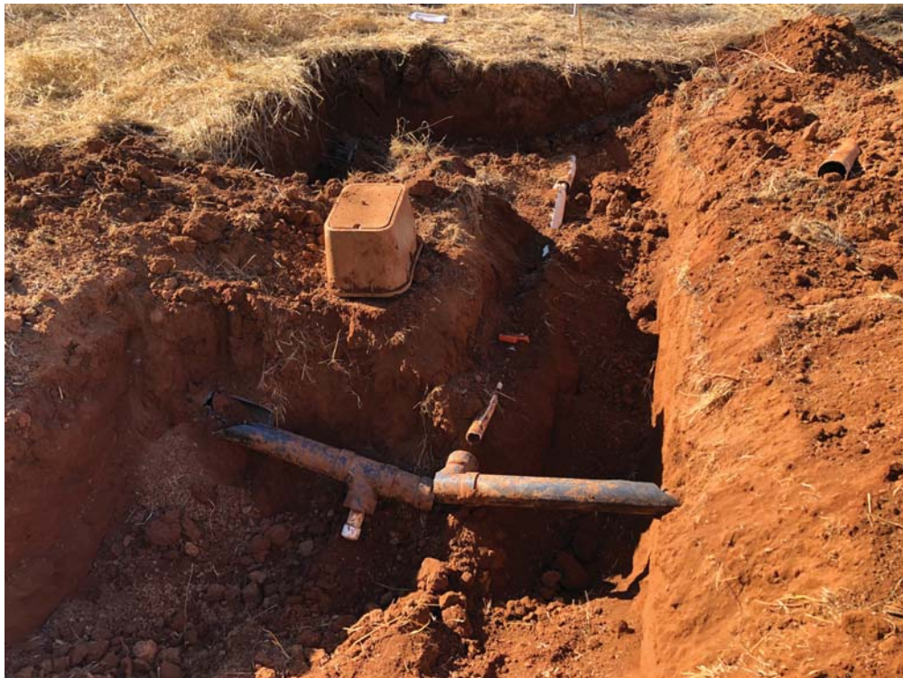
Photo No. 2 Distribution piping exposed in LF1 at the northern margin of Field O. View is looking approximately along contour to the southwest (photo date 8/6/20).
