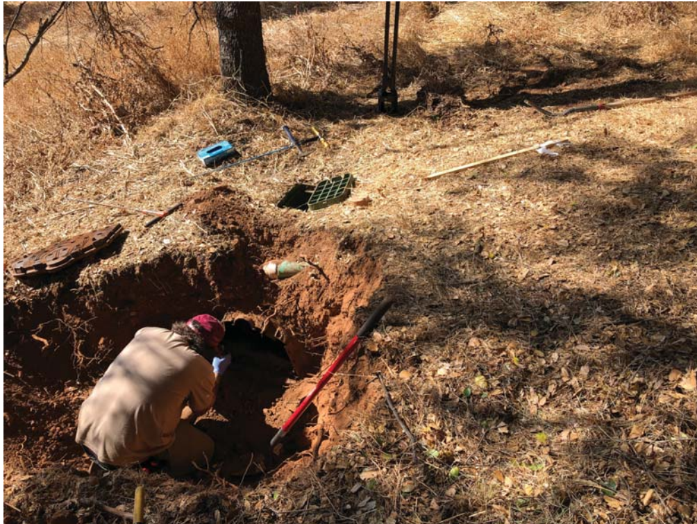
Photo No. 9 Northeast end of Field B, Row 2 infiltrator exposed in excavation LF3. View is looking to the southwest (photo date 8/7/2020).
