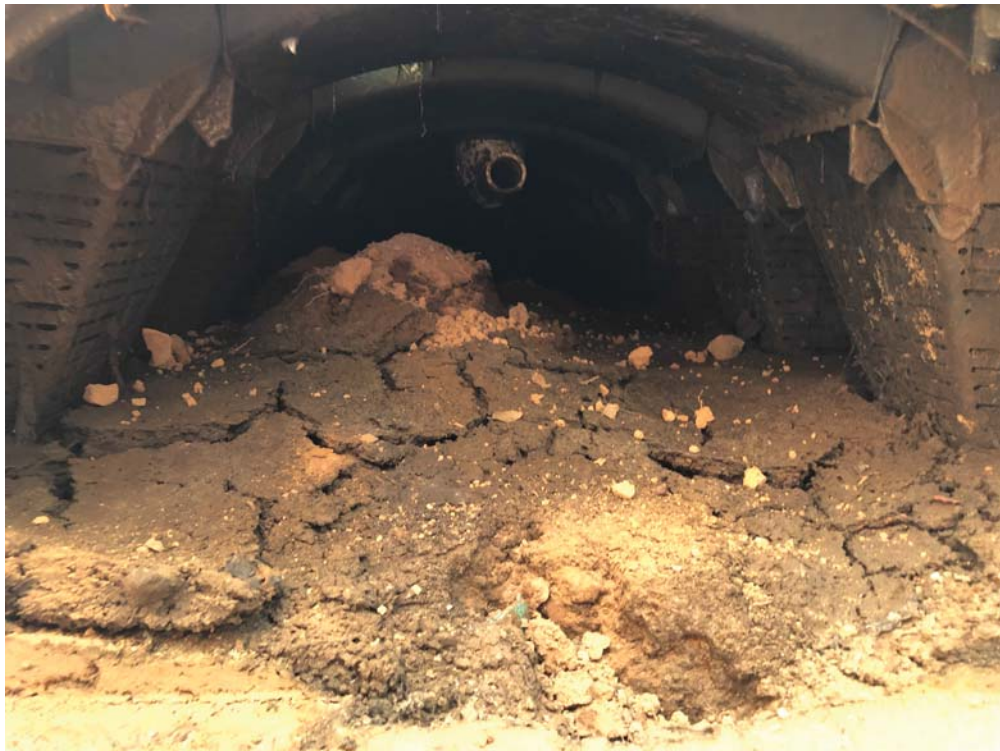
Photo No. 8 Looking into the southwest end of Field B, Row 4 infiltrator (looking to the northeast) (photo date 8/7/2020).
